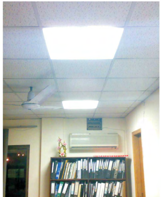
CIMAC lights (40W) installed in an Office
